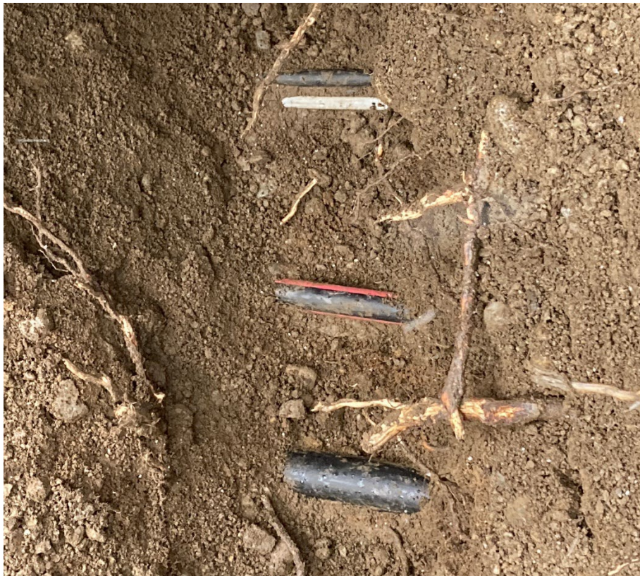
Existing Utility Lines at the East Test Pit. Top to bottom: Astound, Romex, PSE and WSL
