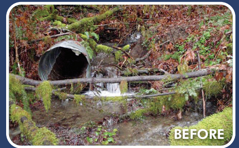
Culvert on Thompson Creek near Rockport creating a passage problem for salmon.
