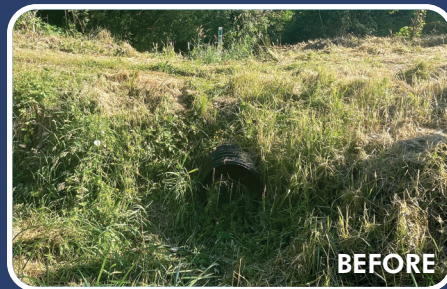
Culverts at Riverfront Park block salmon access in an unnamed creek under a walking trail.
