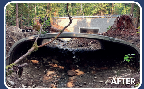
New large culvert reestablishes fish passage on Thompson Creek for salmon and steelhead.
