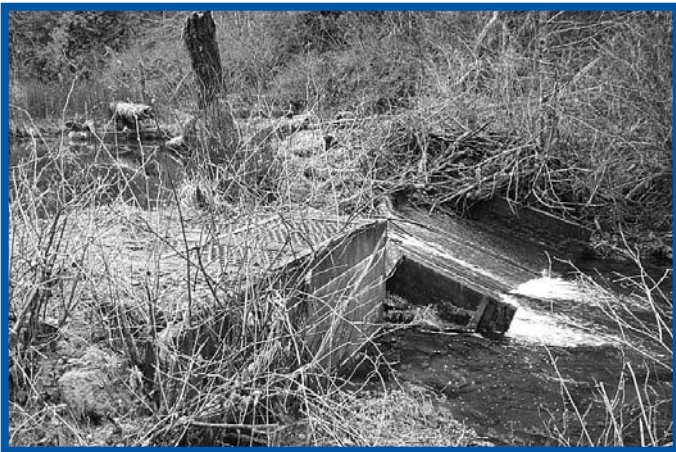
BEFORE: FISH PASSAGE PROBLEM ON SUIATTLE SLOUGH
