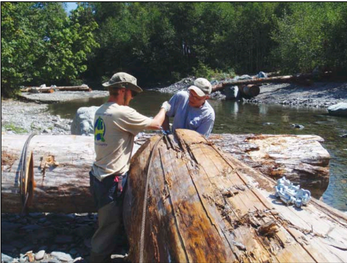
SFEG Restoration Technicians Kyle Koch and Joe George secure log jams in Finney Creek
