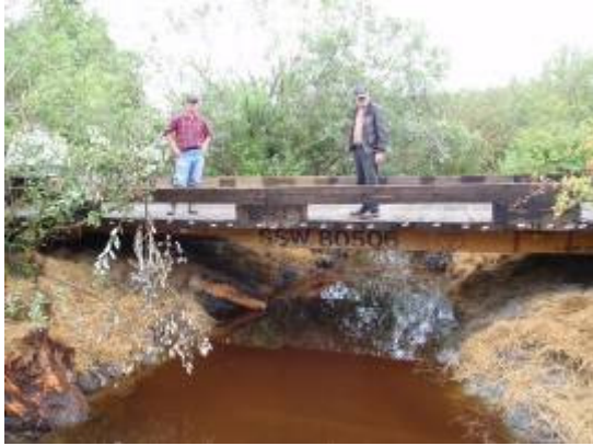
Restoration technician Neil Vargas and resident Bill Sharples atop completed bridge cooperation of local landowners. Funding for the project came through grants from the Salmon Recovery Funding Board and the WDFW's ALEA Volunteer Cooperative Grants.
