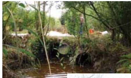
Before impassable culverts on Morgan Creek
